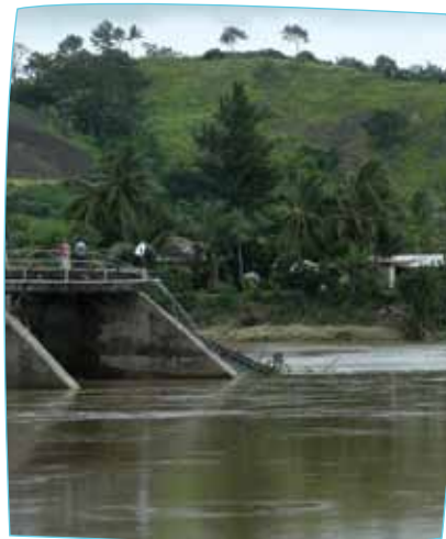
Bridge across the Sigatoka River partially destroyed by severe flooding in January 2009.
