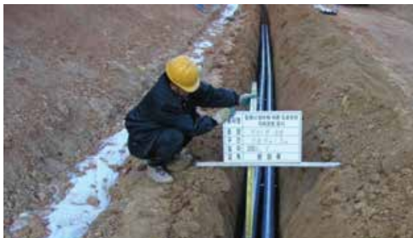
Figure 5.5. Fibre-optic ducts and conduits are placed alongside a highway in the Republic of Korea
